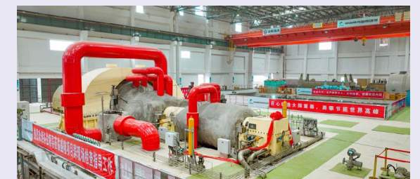
Miniaturized supercritical safe and clean gas-fired power generation technology applied in the supercritical gas-fired power generation project of Guangxi Shenglong Metallurgical Co., Ltd.
